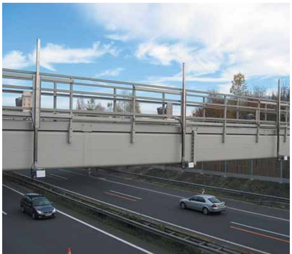
Overhead traffic sensors installed on existing toll station gantry (example: ASFINAG, Austria).
