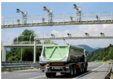
Electronic toll collection – ETC systems
